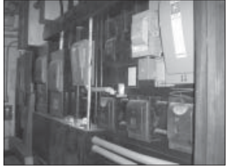
Breaker Room – Power is Controlled.
